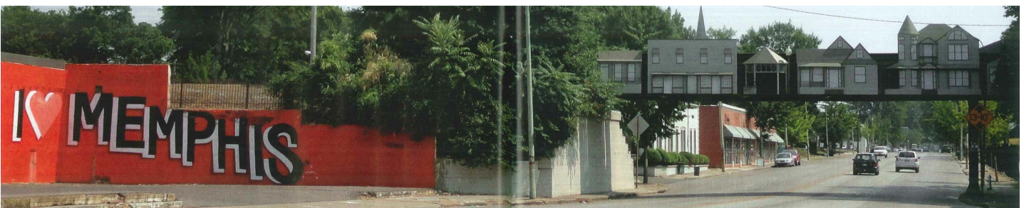
Figure 29 (above): A photo of the railroad viaduct on Amherst Street. A recent visit showed evidence of graffiti, stark conditions, and deteriorated concrete along the retaining walls and traffic median.
