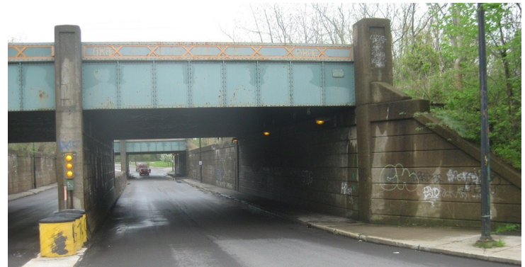
Figure 28 (top): Conditions along the rail just south of Skillen Street. A vandalized, abandoned automobile is at far right.
